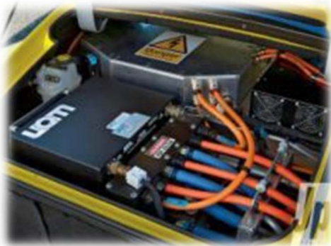
EV Battery Assy
