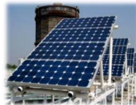
Solar Power Storage
